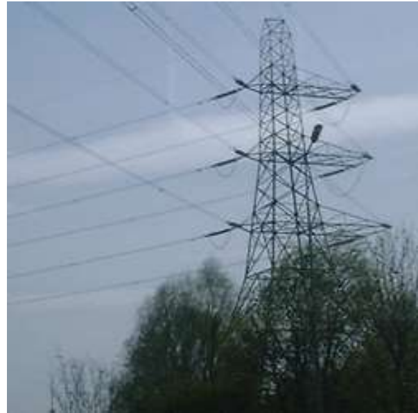
Image 4.2 - Typical tension/angle lattice pylon
