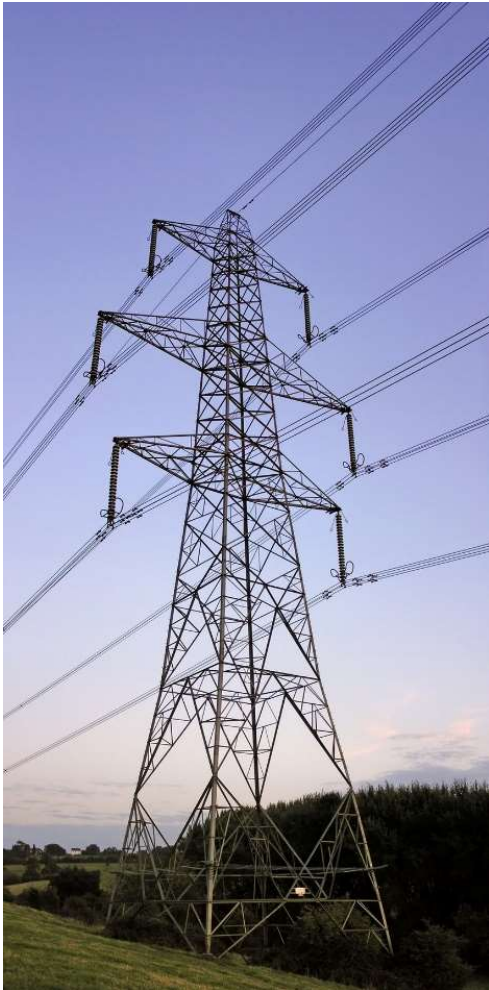
Image 4.1 - Typical suspension steel steel lattice pylon
